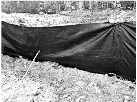
Silt Fence: A BMP used commonly in Pike County to control soil sediment on earth disturbance sites
