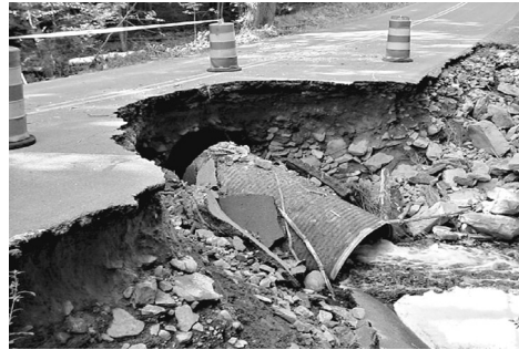
Stormwater damage to community infrastructure
