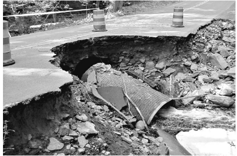
Stormwater damage to community infrastructure
